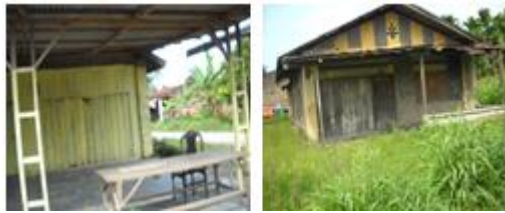
Figure 2: Physical State of the Building
