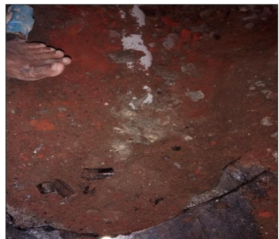
Figure 5: Bricks used instead of Waterproof membrane
