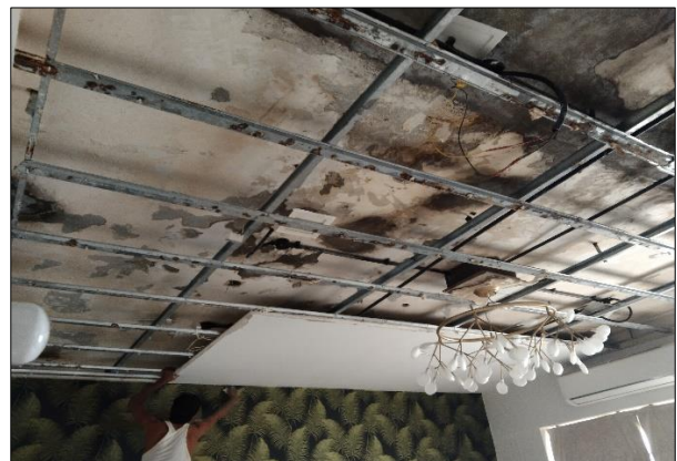
Figure 1: Condition of the Subject Ceiling on Level 1
