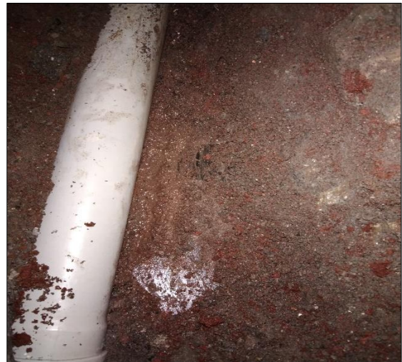
Figure 5: Water near Underground Pipes
