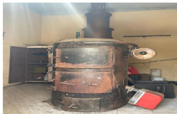
Figure 4: Shows Omdurman Maternity Hospital incinerator
