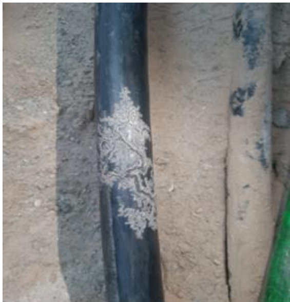
Figure 4: Bonding Cable Sheath Fault
