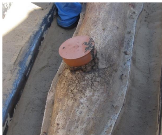
Figure 6: Sheath Fault in Cable Joint
