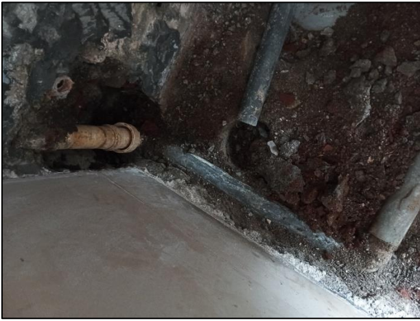
Figure 4: Rusted underground GI pipes
