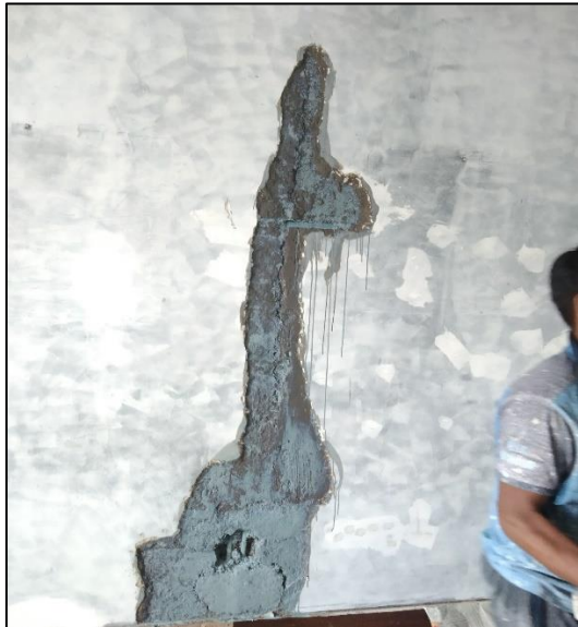
Figure 1: Seepage near Concealed electrical wiring
