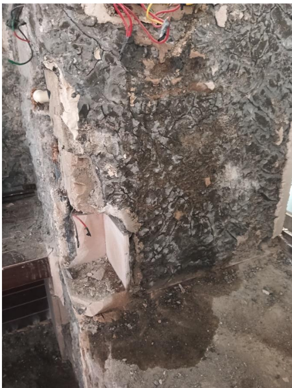
Figure 7: Water Seeping into the concealed switchboard from the duct area
