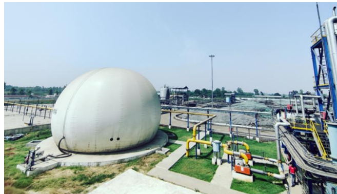
Figure 4: Biogas plant storage
