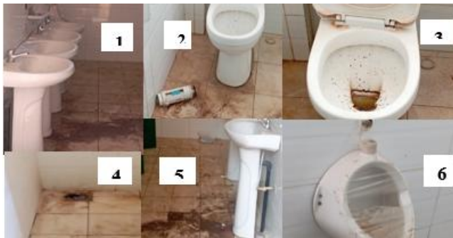
Plate 1: Sanitary facilities in poor working order or poorly maintained
