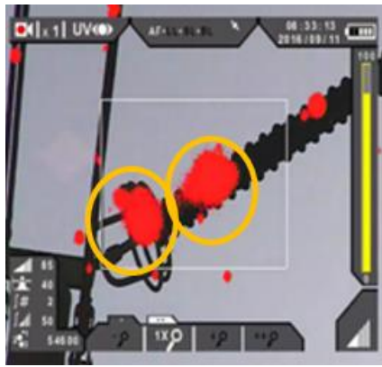
Figure 3: Defective Insulator with High Corona Discharge
