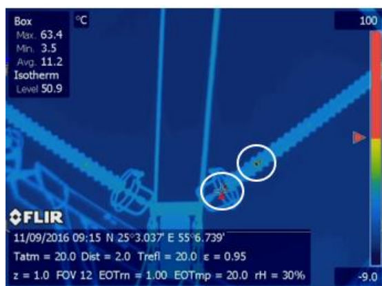
Figure 4: Defective insulator identified using IR Camera
