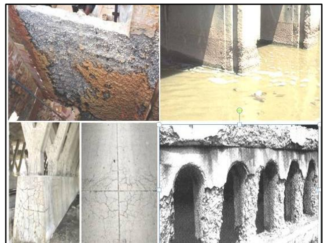
Figure 1: Deterioration of concrete structures (anticlockwise from top left) (Chemical reactions, Aggressive water attack, Freeze and thaw process and alkali silica attack)
