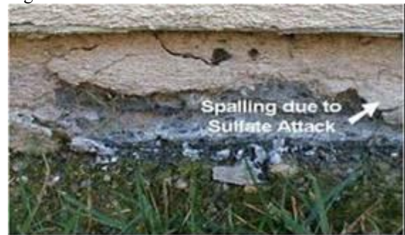
Figure 2: Spalling due to sulphate attack
