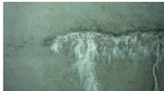
Figure 3: Leaching of concrete
