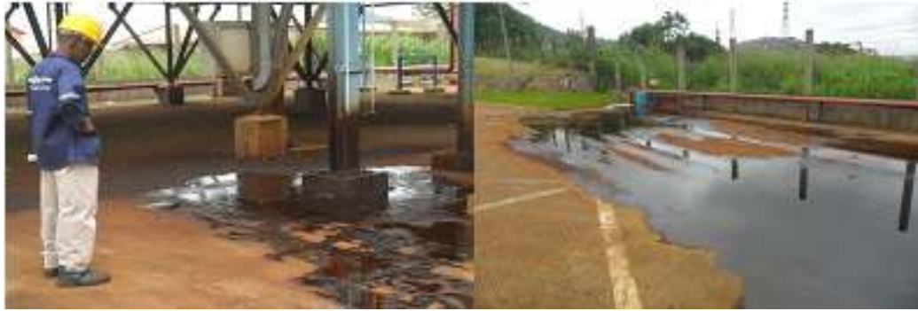
Figure 12: Dumping of products in the receiving environment due to a leak in the coolant-oil heat exchanger coming out of the bleed (TPO)
