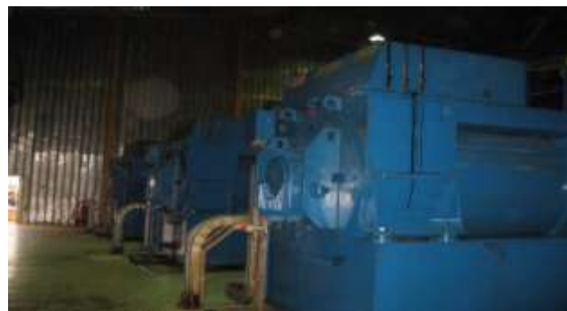
Figure 1: Engine room at OYOM-ABANG I
