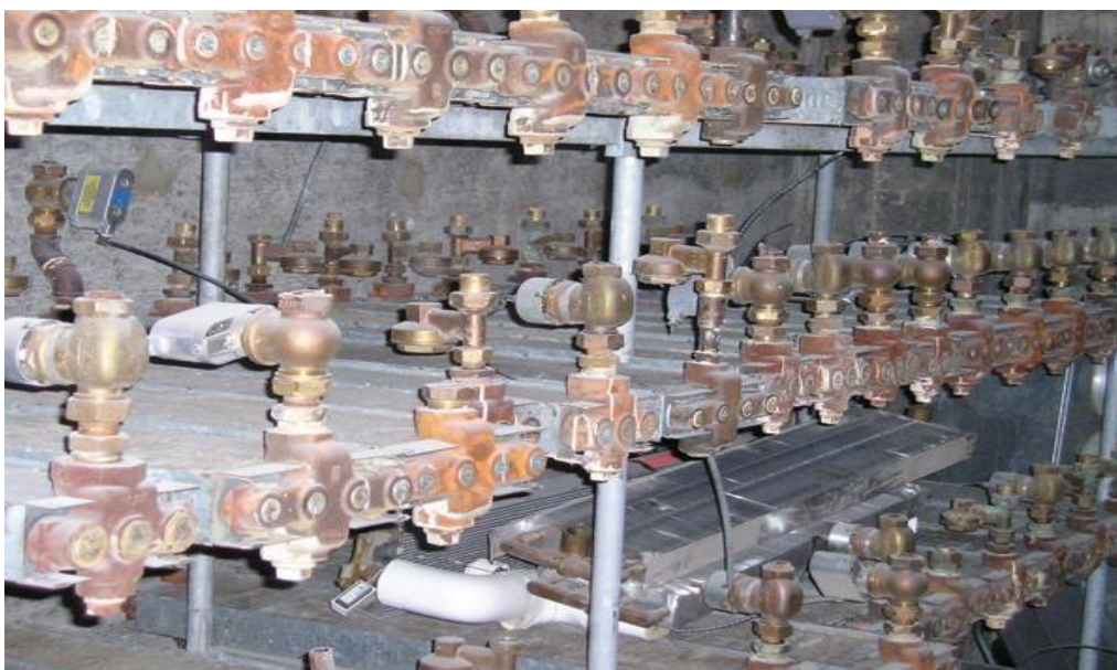
Figure 1: Example of an Old Buildings Hold Retrofit Challenges
