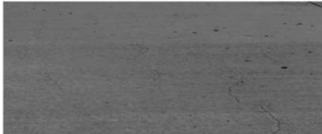
Figure 1: Plastic shrinkage in a Bridge deck
