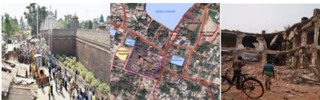
Figure 7 (a), (b), (c): The demolition around the Lingaraj temple, for renovation; during 3/20. 2020
